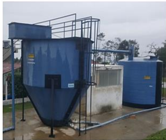
Figura 6. Planta semicompacta Coovesur
