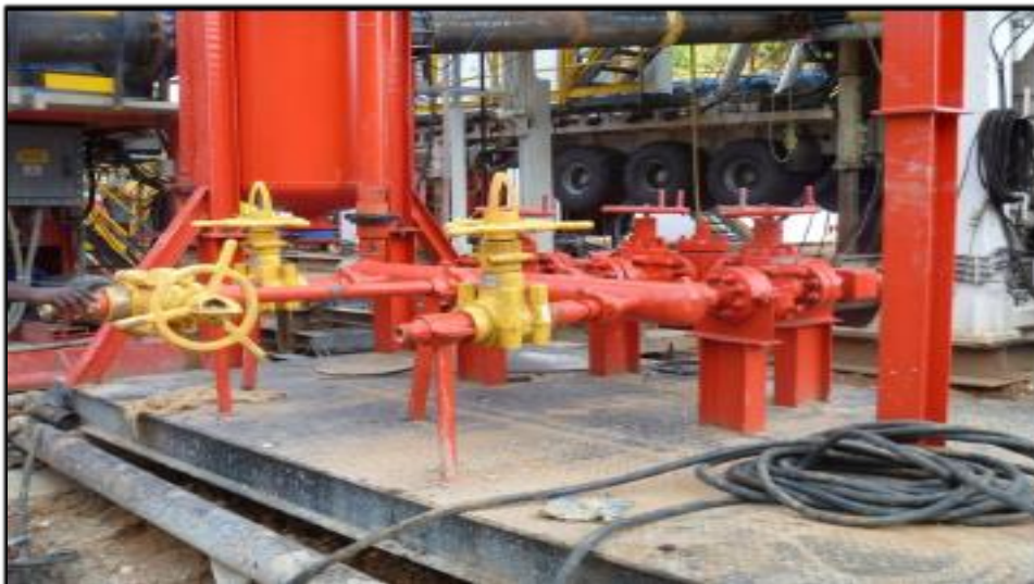
Figura 7. Choke manifold 3 1/8'' x 5M
