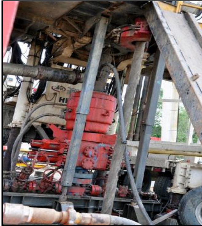
Figura 5. BOP stack de 13 5/8'' x 5M RIG 51
